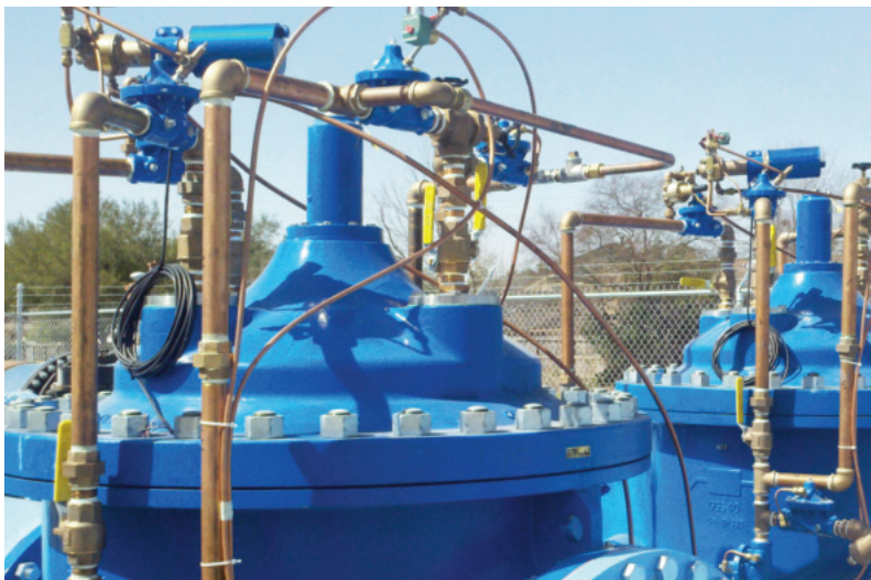
Meter Station/ Point of Custody Change: Three 30-inch Pressure Reducing/Pressure Sustaining Valves
