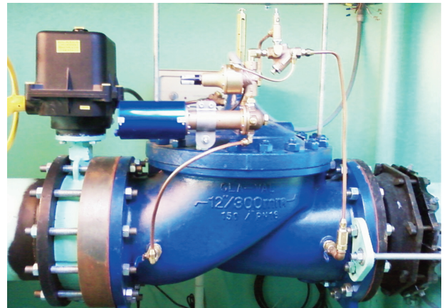
Underground Vault: Pressure Reducing/ Pressure Sustaining Valve feeding nearby community and elevated storage tank two miles downstream of the electronic control valve.
