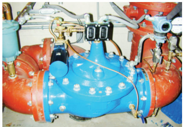
Reservoir Site: Pressure Sustaining Valve for Reservoir Filling.
