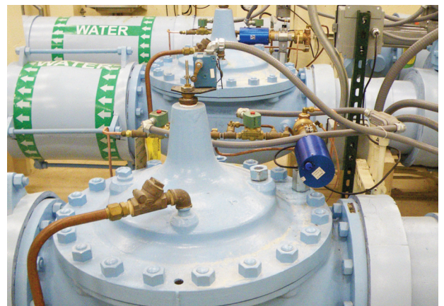
Water Treatment Facility: Pressure Reducing Valves capable of easy adjustment for demand variations.
