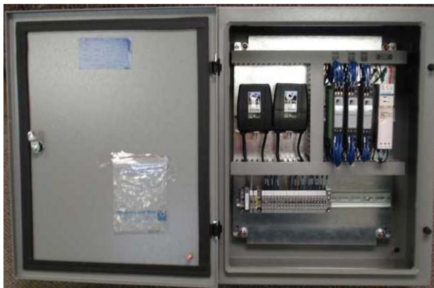
Figure 6 - PRV Control Panel & Wiring Strip
