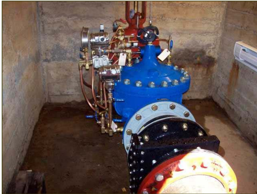
Figure 5 - Donlands & Aldwych Flow Modulating PRV Installation
