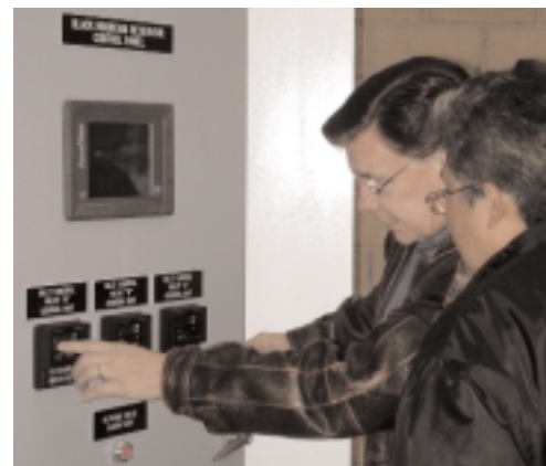
Electronics Products Division Manager Don Compton configures and tunes each Cla-Val 131VC-3 controller.
