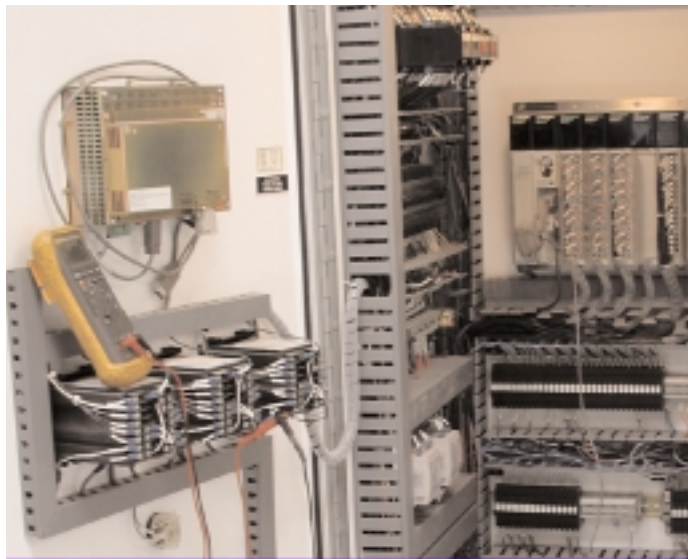
Cla-Val 131VC-3 controllers mounted onto panel (on left) are wired into SCADA PLC inside cabinet. Startup checks are made by Cla-Val personnel to ensure proper operation.
