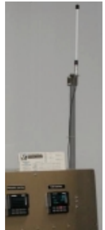
RTU radio antenna
