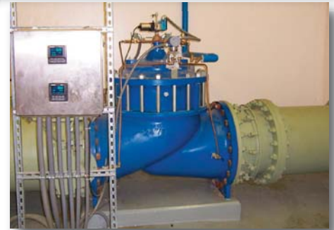
Modulating Level Control with Metering
