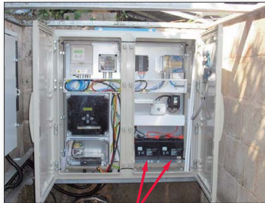
Two 12 Volt batteries for 24 VDC total
