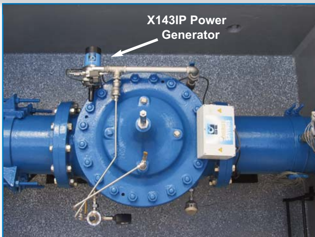
Typical Installation: Pressure Reducing Valve Station X143IP providing power to operate electronic valve controls, data logger, pressure transducers and the Cla-Val X144 e-FlowMeter™
